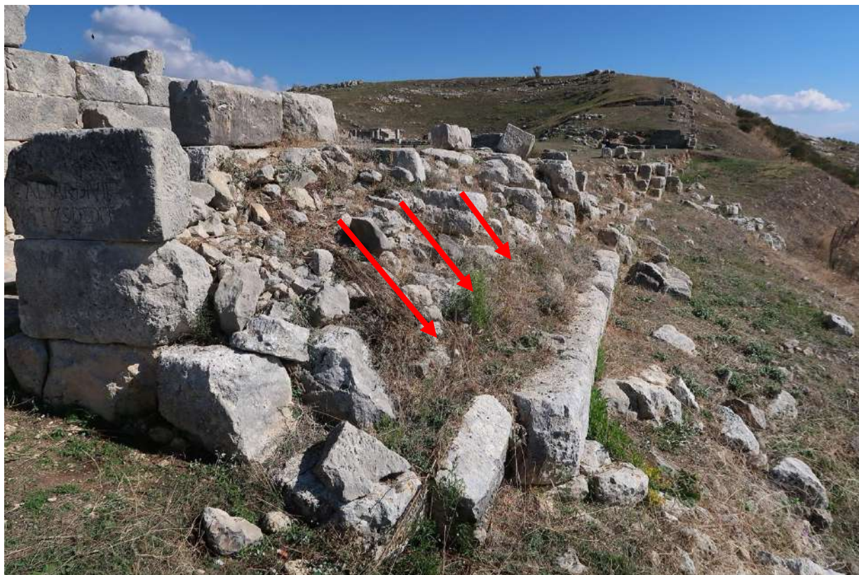
Figure 13 Uncontrolled slippage of masonry blocks, potentially hazardous for both conservations and safety reasons.
