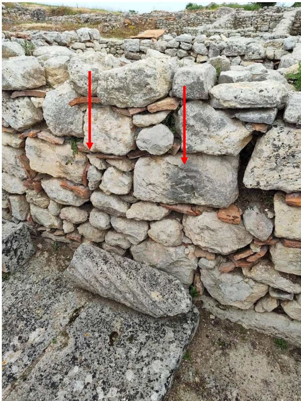
Figure 15 Wall crest deformations and structural failures; ineffective stabilization with improper infill (pottery fragments).
