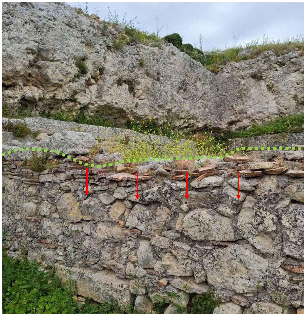
Figure 93 Wall crest deformations and structural failures; ineffective stabilization with improper infill (pottery fragments) and scattered, poorly executed repointing with cementitious mortar.
