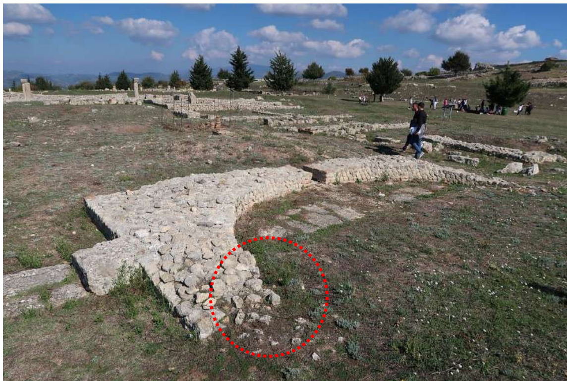
Figure 8 Erosion of cementitious joint repointing, facilitating vegetation growth and loss of archaeological legibility.
