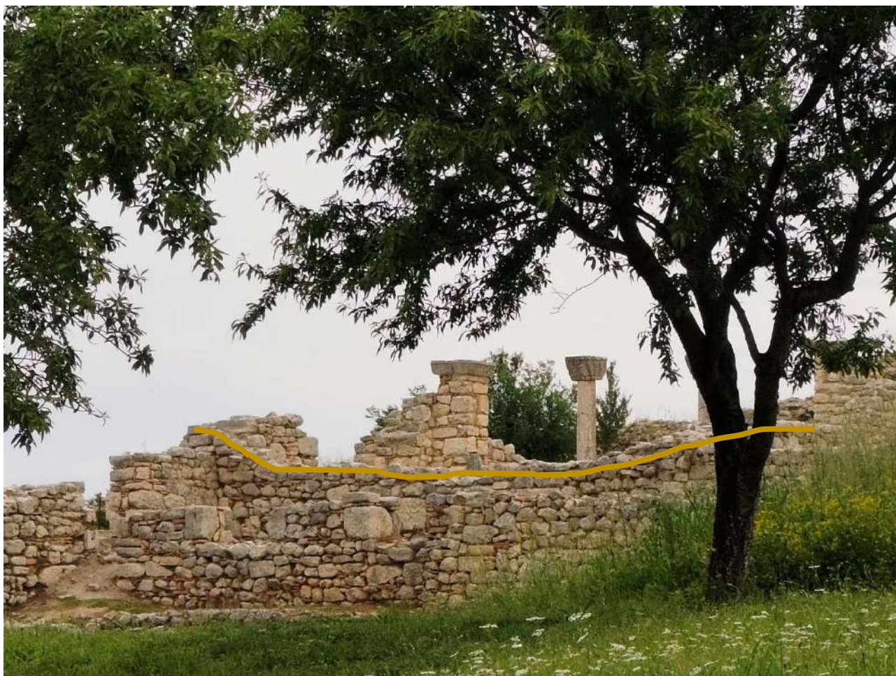
Figure 81 Absence of a protective casings to stabilize the wall crests and prevent settlement, material loss, and vegetation growth.
