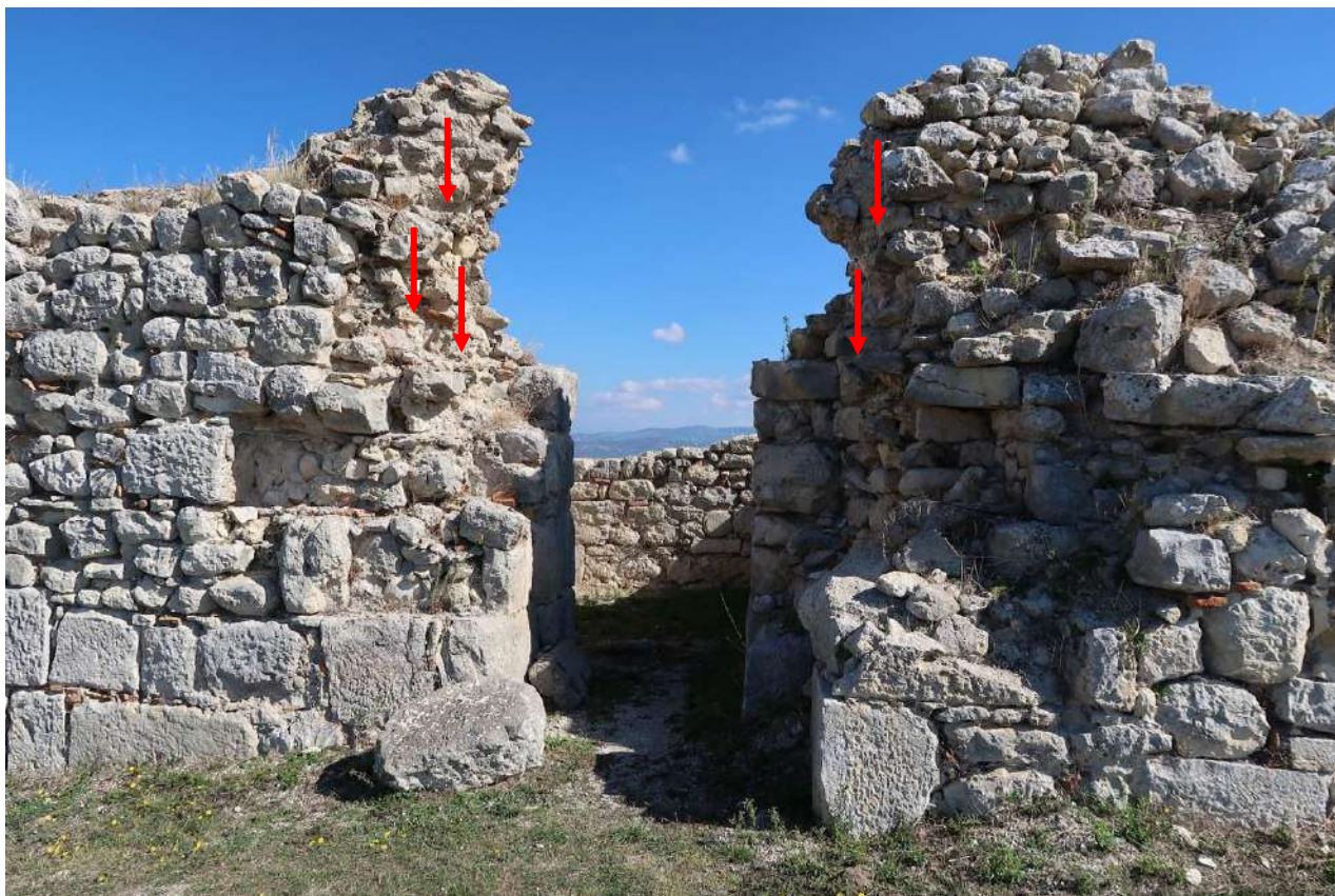
Figure 29 Risk of wall-crest collapse and structural failure of the portal as shown by the concrete lintel replacements already arranged along the openings of the walls and towers, posing a hazard to visitor circulation.
