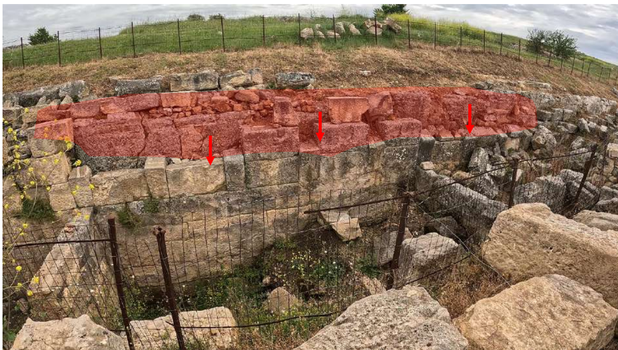
Figure 10 Structural failures of the blocks in the retaining walls of the cistern, caused by soil pressure and slippage. Cisterna
