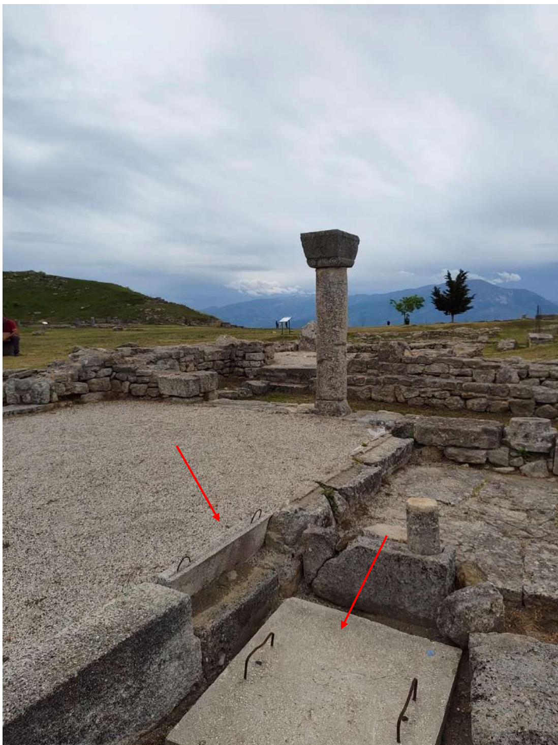
Figure 33 Concrete blocks used as infill for missing areas and for protection, temporary in appearance and inconsistent with both their intended function and the site's aesthetics.
