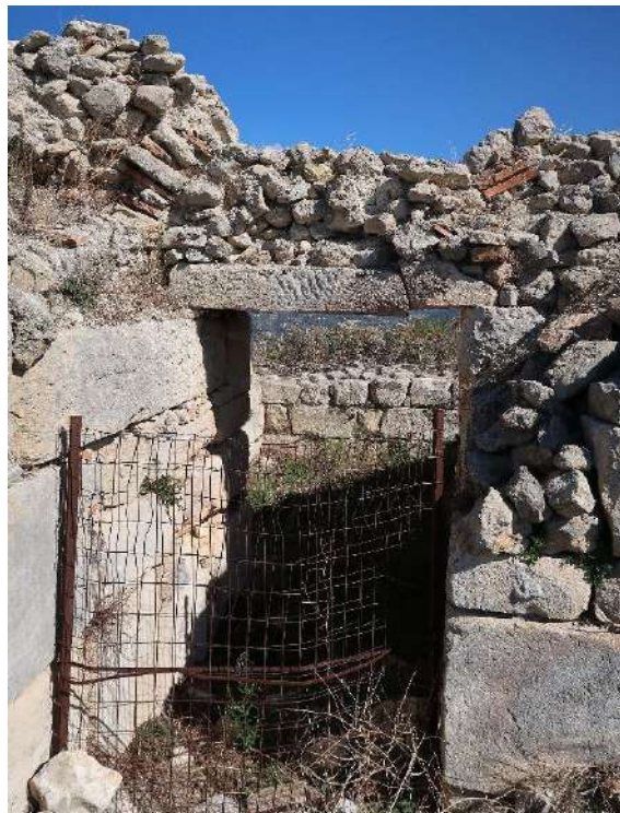
Figure 10 Critical cracks of the lintel in the entrance of the Tower X
