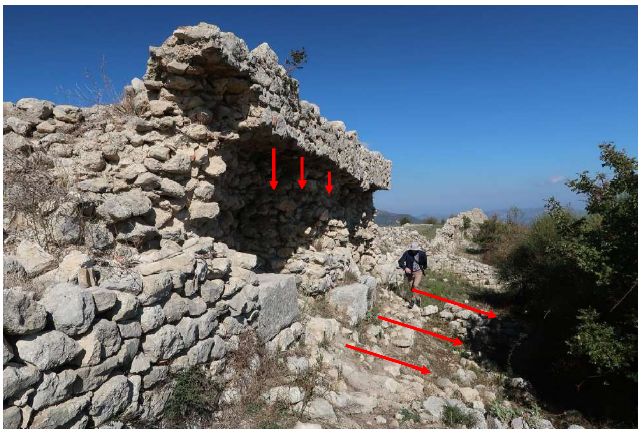
Figure 27 Significant loss of masonry blocks, posing hazards to both conservation and safety, possibly due to anthropogenic activity, and facilitating vegetation rooting further endangering the walls' stability.
