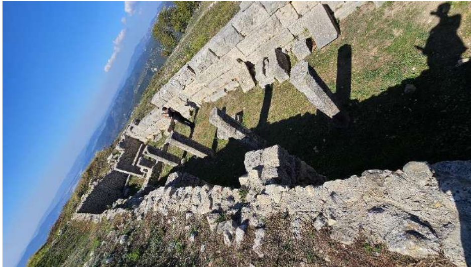
Figure 9 Arsenal after restoration. A risk of colonnades overturning has been observed
