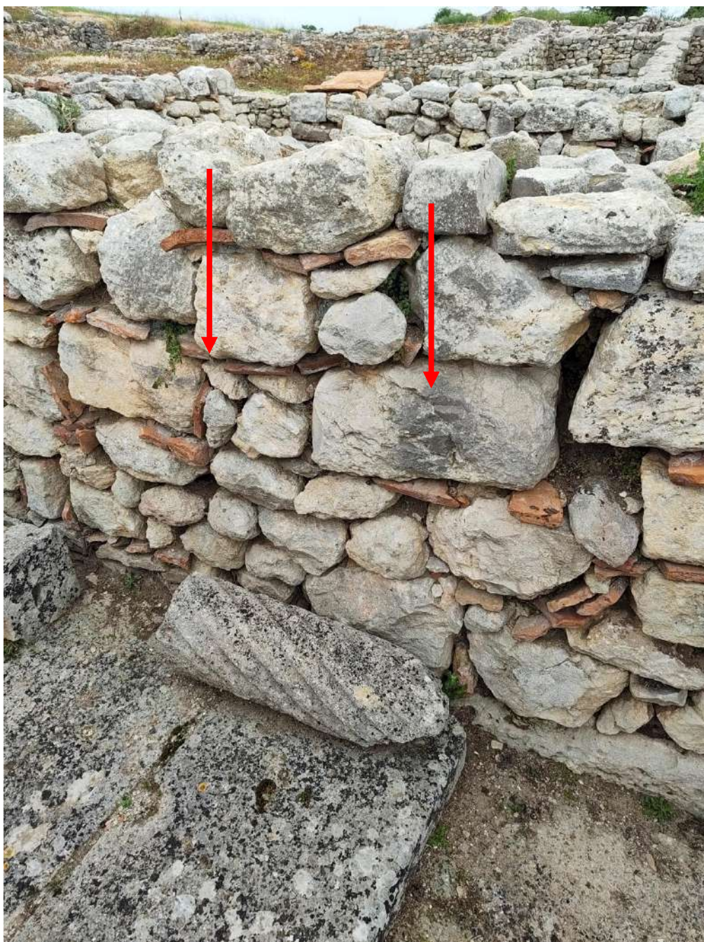
Figure 20 Wall crest deformations and structural failures; ineffective stabilization with improper infill (pottery fragments).
