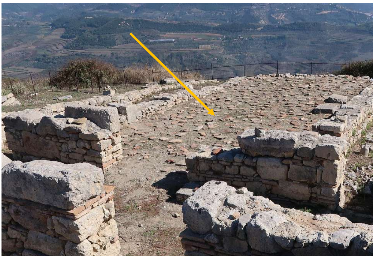
Figura 104 Resettlement and compaction of the soil with improper infill (pottery fragments), facilitating weeds growth.
