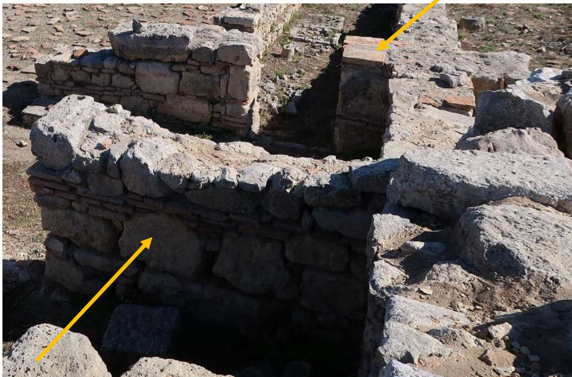
Figure 7 Erosion of wall crests and deterioration of cementitious joint repointing and stabilization with improper infill (pottery fragments). Basilica E
