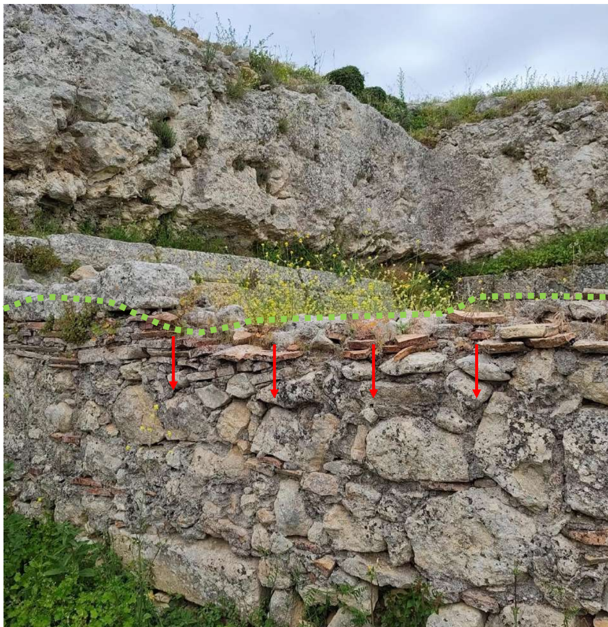
Figure 17 Wall crest deformations and structural failures; ineffective stabilization with improper infill (pottery fragments) and scattered, poorly executed repointing with cementitious mortar.
