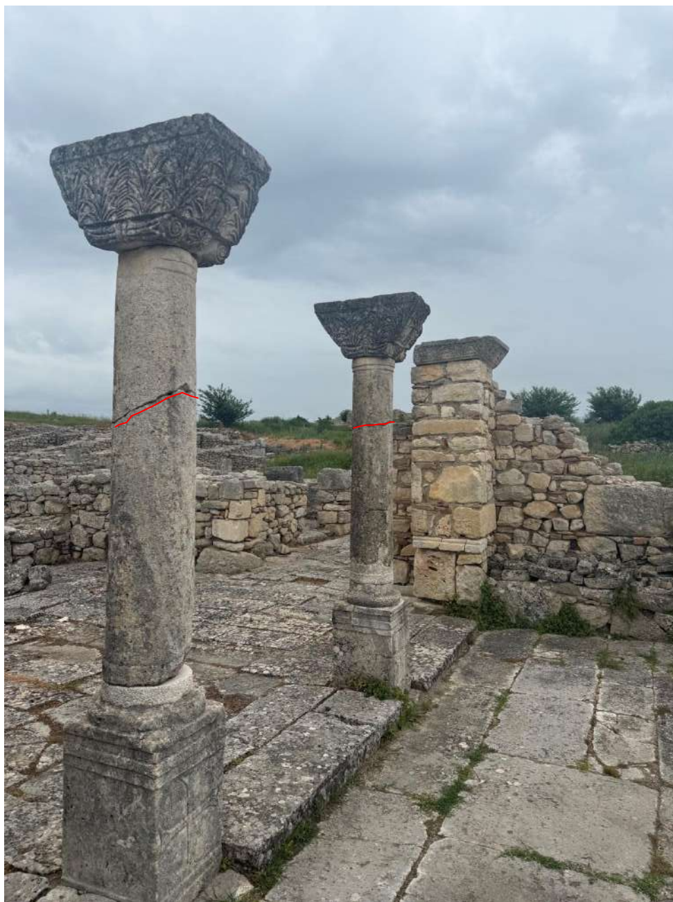
Figure 19 Deep fractures visible in the columns of Basilica B.
