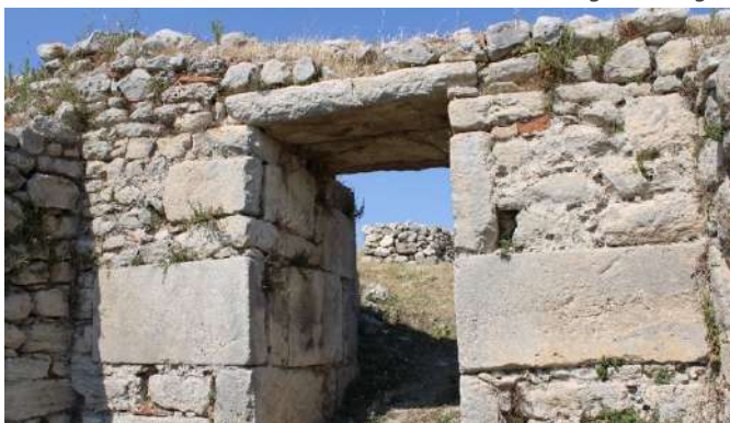
Figure 87 The tower's U gate. The cracked architraves
