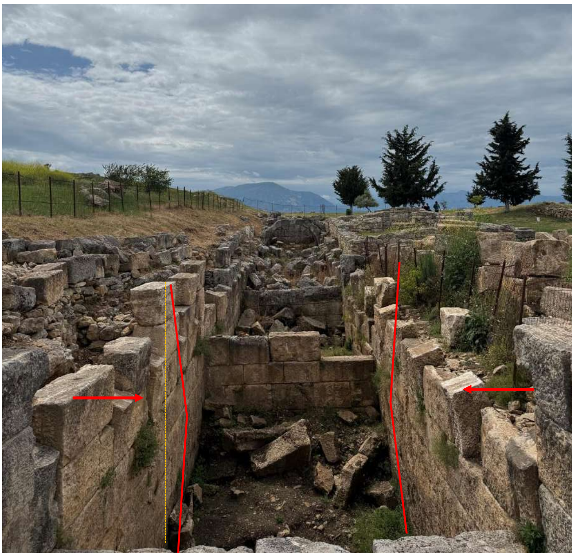
Figure 16 Structural failures of the blocks in the hypogean retaining walls of the cistern, caused by soil pressure and slippage.
