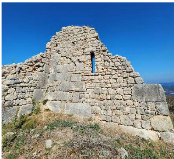
Figure 4 Exterior frontal view of the Victorious Wall located in the Section T-U, highlighting diagonal cracking, indicating the risk of imminent collapse
